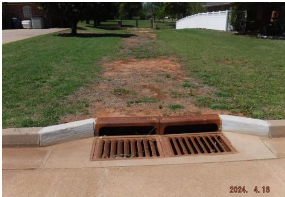
Figure 5: VIEW FROM PONDRIIDGE RD. OF THE CATCH BASIN AND PIPE ALIGNMENT ACROSS THE MARSHALLS PROPERTY
